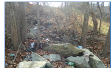
Figure 4-1. Drainage culvert with accumulated trash
